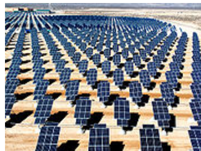
Nellis Solar Power Plant, the largest photovoltaic power plant in North America
